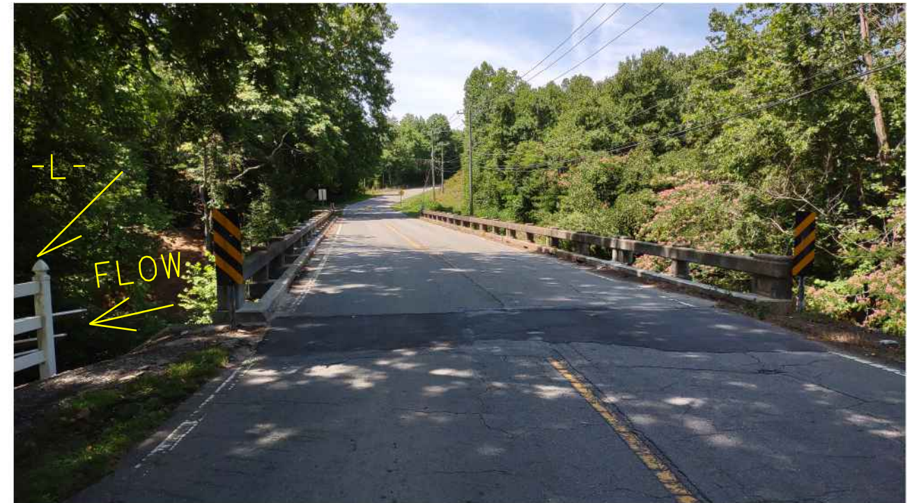
PHOTO #2: NORTH EAST END OF BENT 2 SIDE OF EXISTING BRIDGE LOOKING SOUTHWEST (DOWNSTATION)
